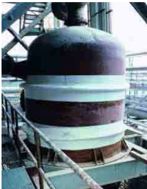
Chlorine dioxide tank installed in 1966
